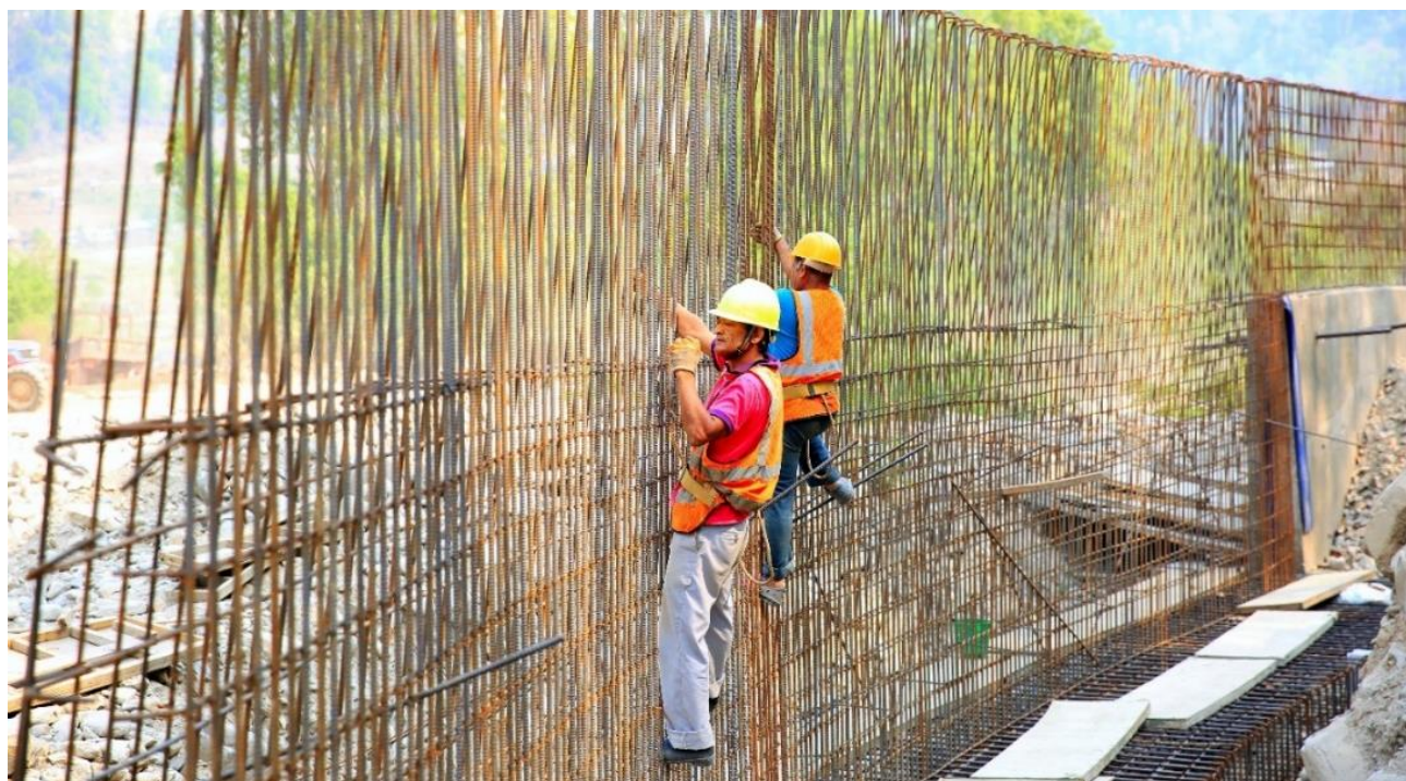
Figure 3: Workers constructing gabion wall to prevent seasonal flooding. Photo credit: UNDP Nepal
