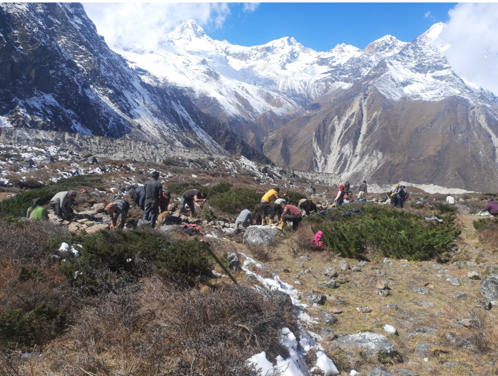
A 1300m trekking foot trail has been constructed in Taplejung that passes through rugged mountain terrain at an altitude of 4200-4700 m above sea level. The trail is one of hundreds of small tourism infrastructures constructed under Sustainable Tourism for Livelihood Recovery Project, a joint initiative of Nepal tourism Board and UNDP Nepal. Photo: STLRP/UNDP Nepal
